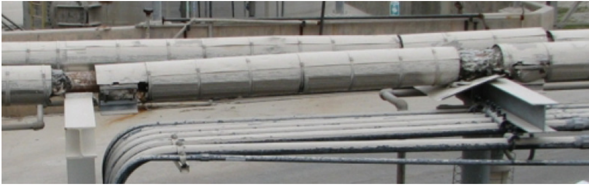
Figure 1. Example of uncontrolled expansion.
