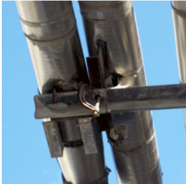
Figure 2. Example of uncontrolled expansion and lack of guides to avoid buckling and lateral movement.
