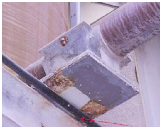
Figure 3. Support at tipping point due to uncontrolled expansion.
